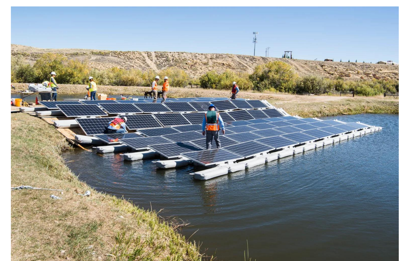
Example of 'floatovoltaics' in Colorado
